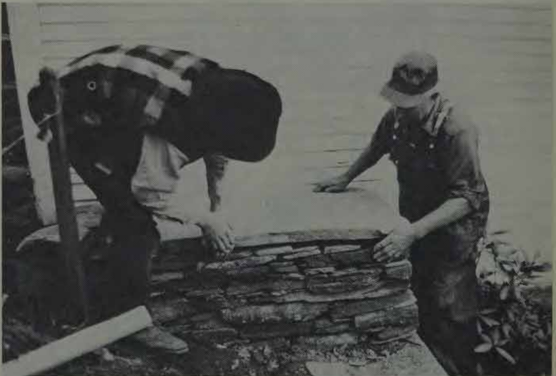
A topping stone is placed on a corner, carefully pre-built to accommodate the stone's slight arch.
