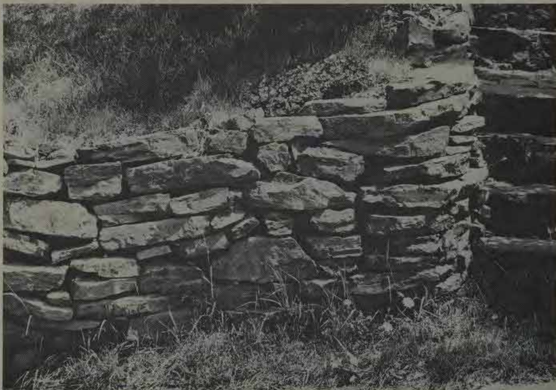
A supply of fairly good stones is put together so as to invite problems. Note the excessive run to left of steps.
